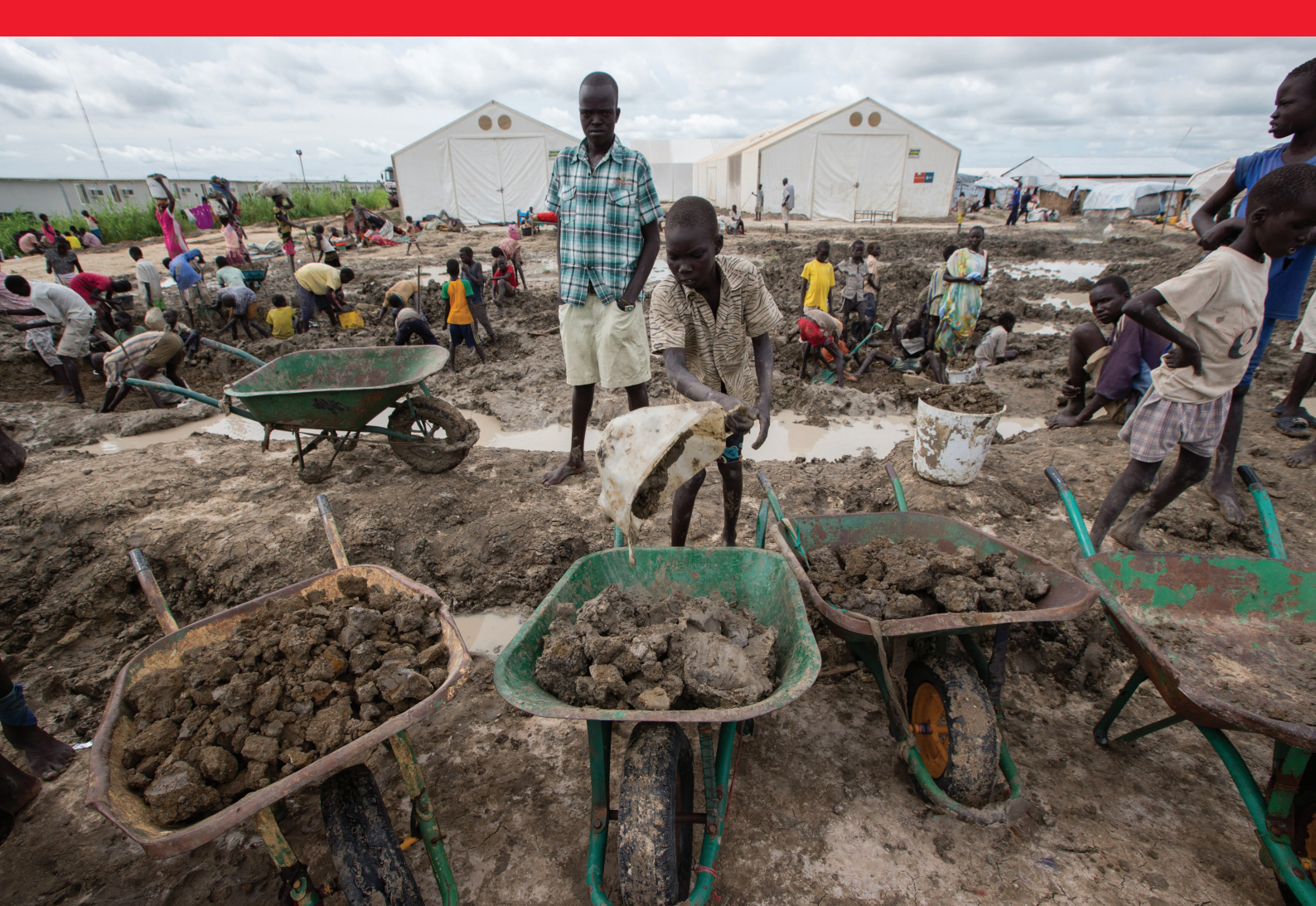
A boy fills wheelbarrows with dirt to build walls in the Protection of Civilians (POC) site near Bentiu, Unity State
