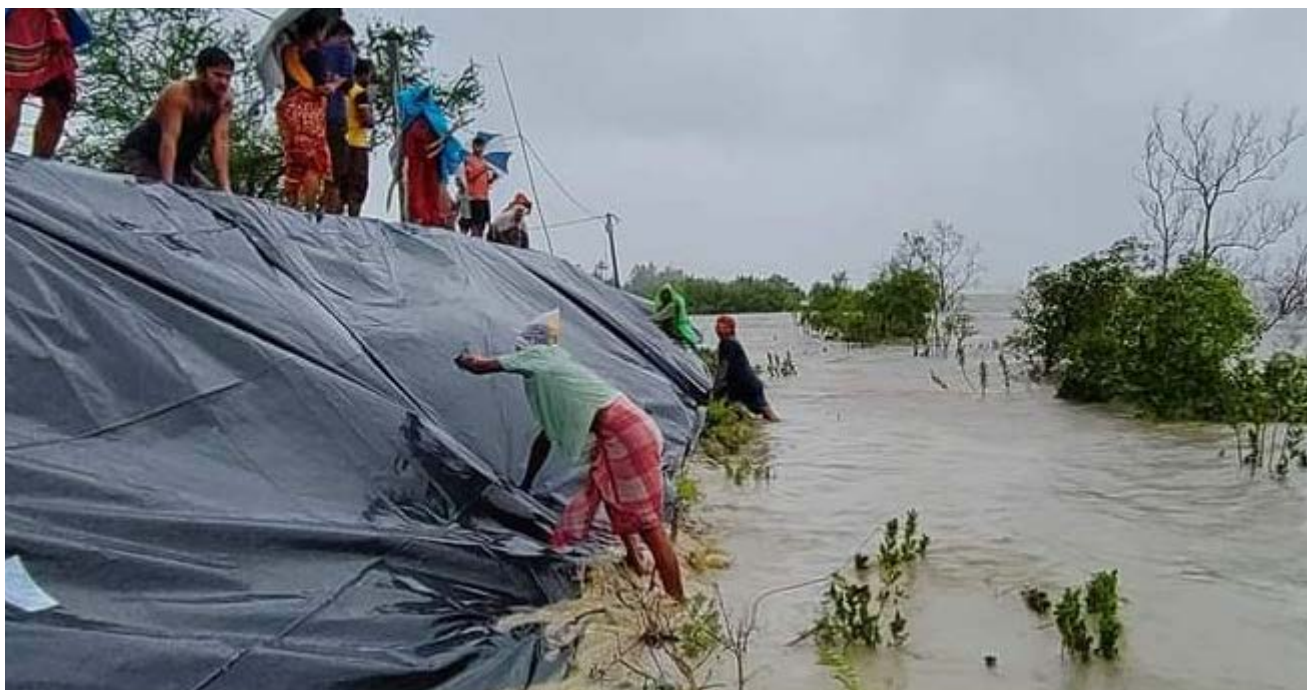
A group of community members and disaster management volunteers work to reinforce an embankment in a flood-affected area of the Gosaba block. Credit: Bappi Sarkar, VDMF member
