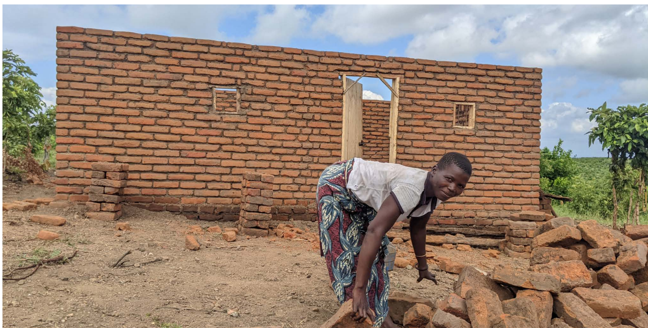
Esnart constructs her new home in Chataika Village after climate-induced displacement, using unconditional cash transfers from GiveDirectly to purchase the building materials. Credit: GiveDirectly
